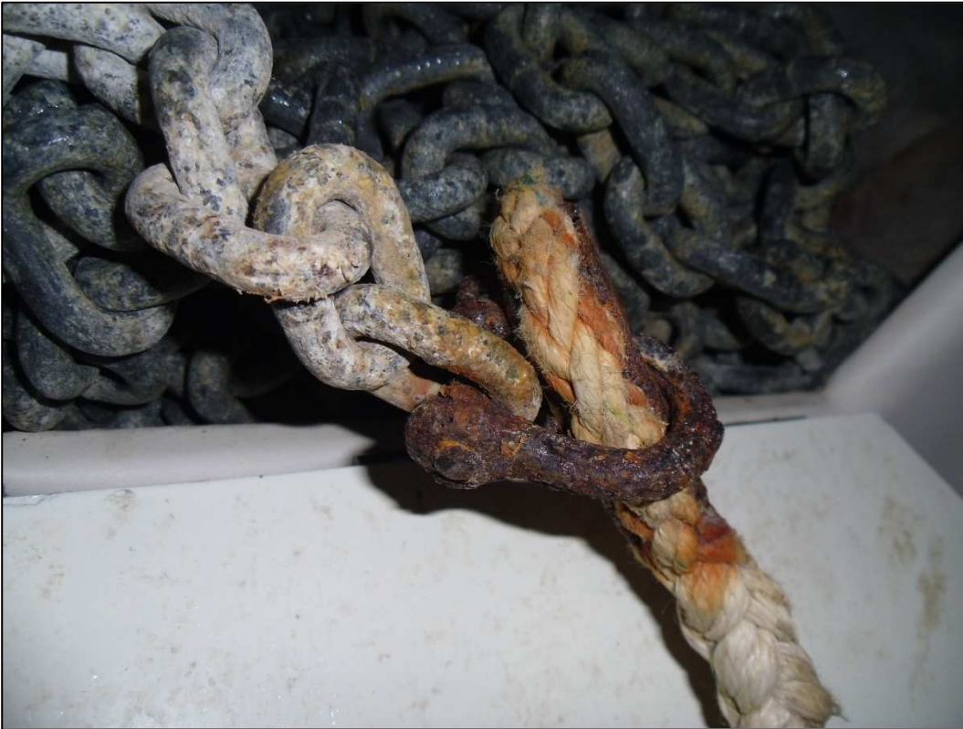
Fig.3 – chain bitter end to rope connecting shackle is corroding.
