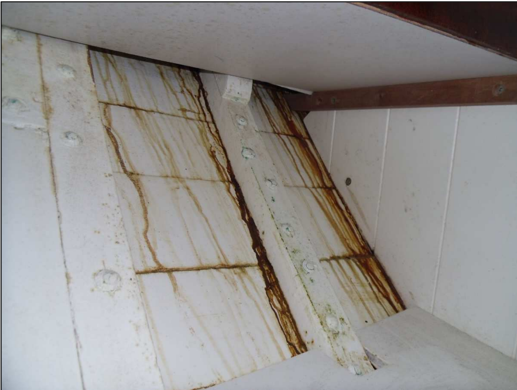
Fig.5 – example of weeping from the structure / planking.
