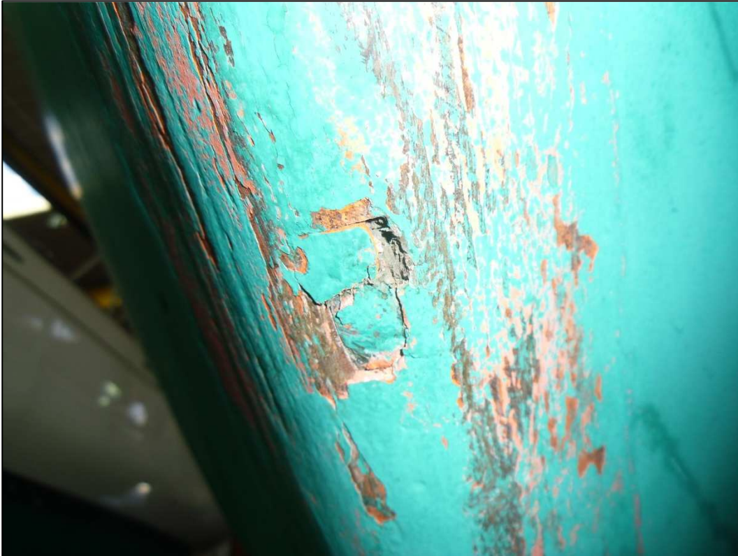
Fig.2 – small area of damage to the bow stem below the waterline.
