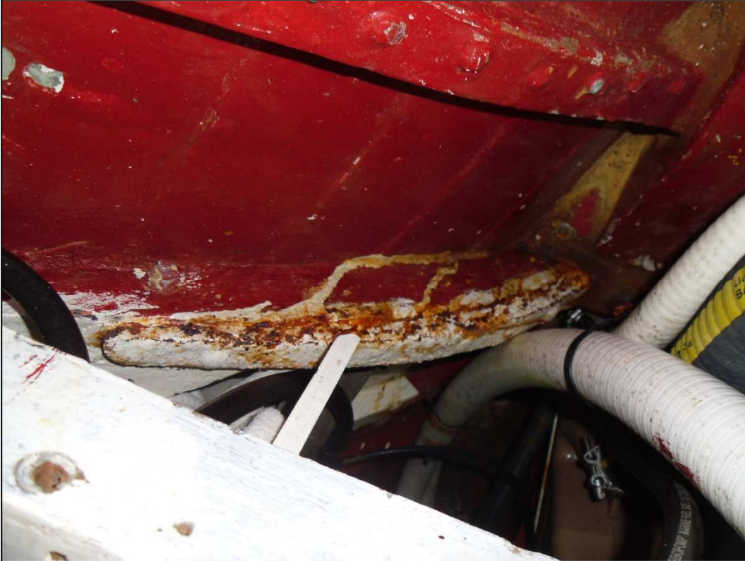
Fig.4 – signs of corrosion and weeping from the lazarette iron floors.
