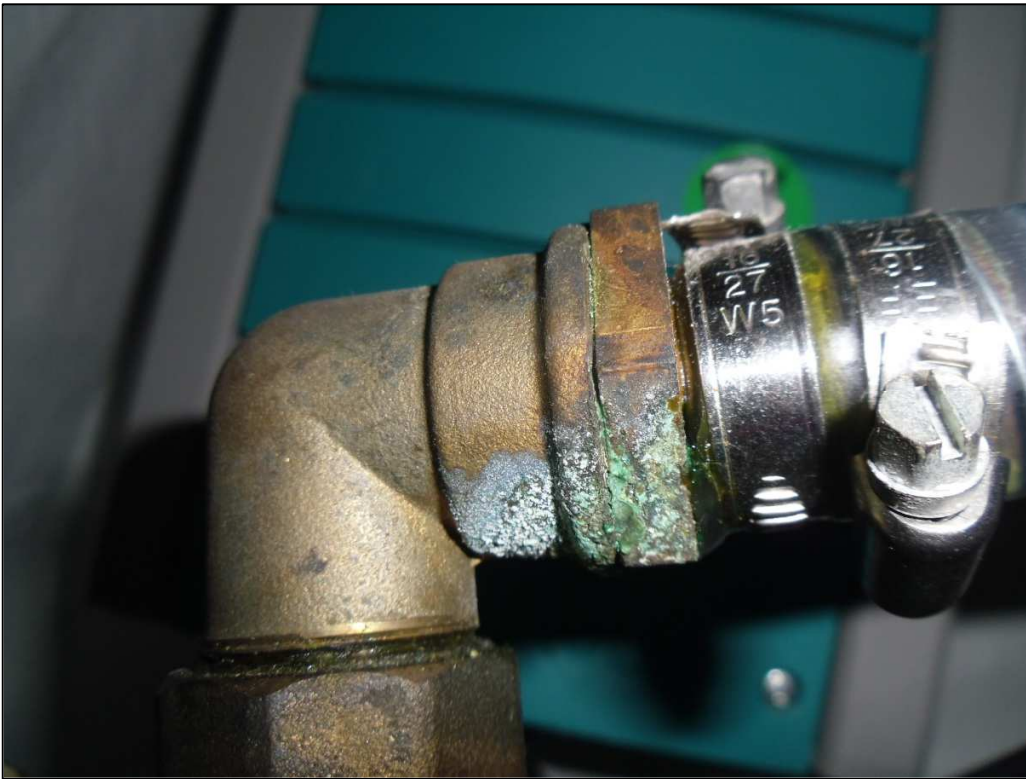
Fig.5 – corrosion / leak from the toilet inlet seacock to hose join.
