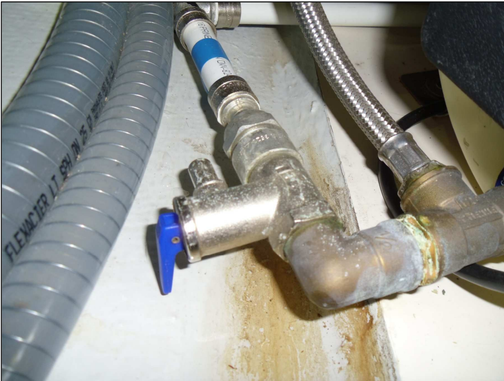
Fig.4 – leak from the pressure relief valve or elbow connection to the T piece.
