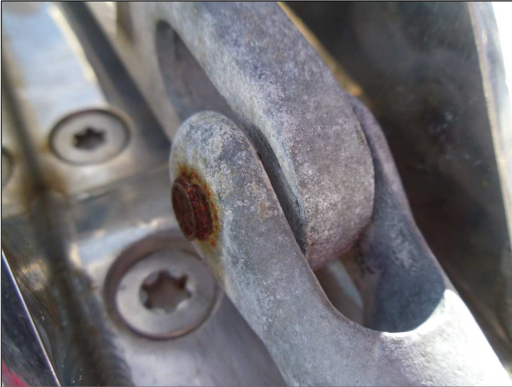
Fig.3 – anchor to chain connection fitting is showing corrosion.
