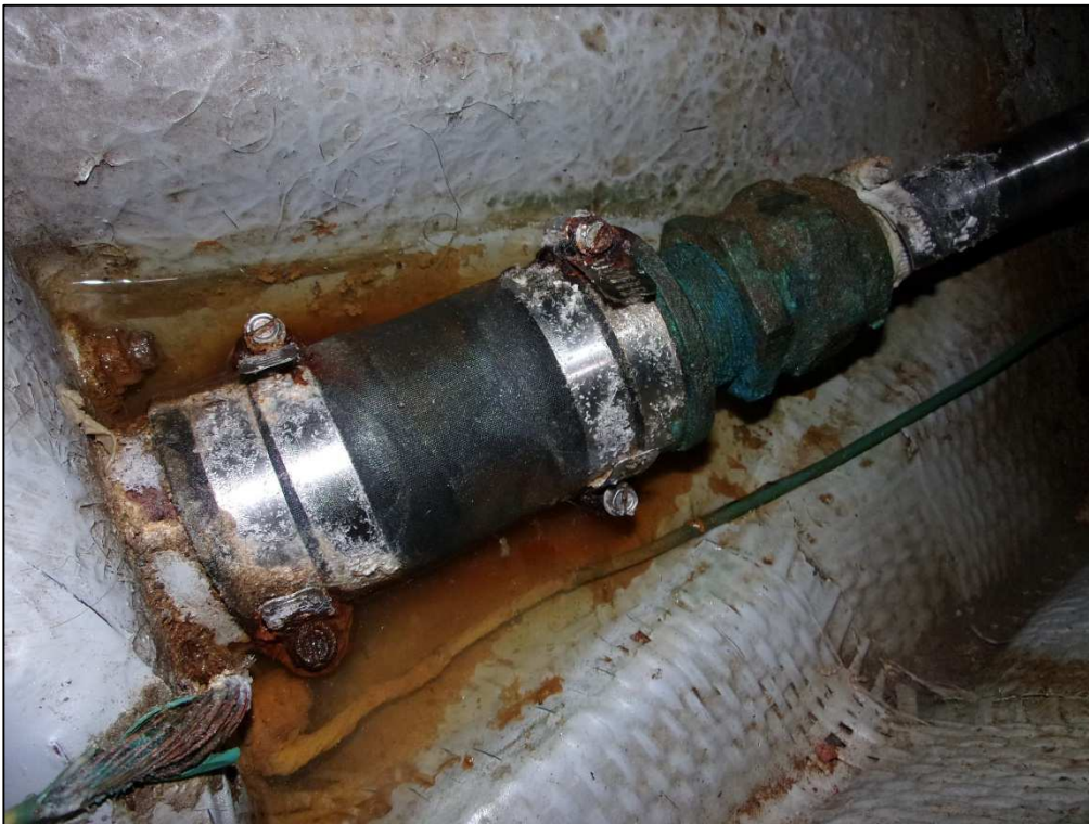
Fig.1 – stern glands showing corrosion to stiffing box and fixings.
