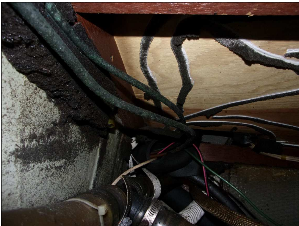
Fig.3 – copper fuel pipes with surface corrosion.
