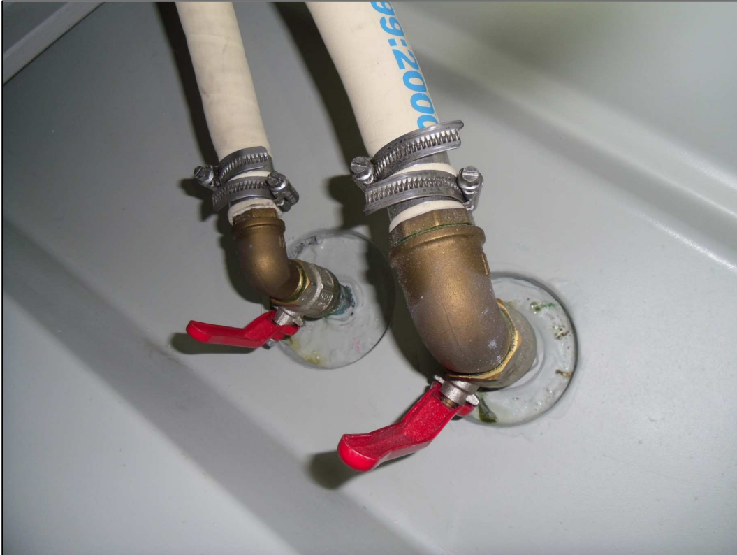
Fig.3 – both toilet seacocks showing some small droplets of salt water.
