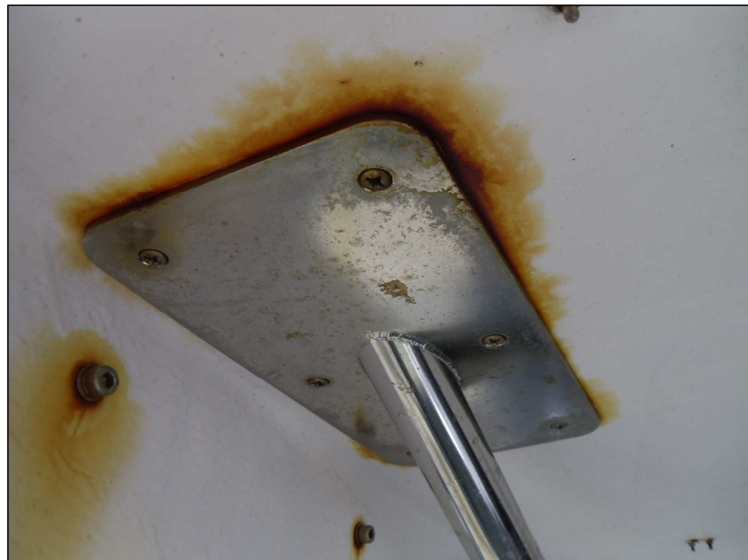
Fig.1 – corrosion staining to the platform securing bolts and support brackets.
