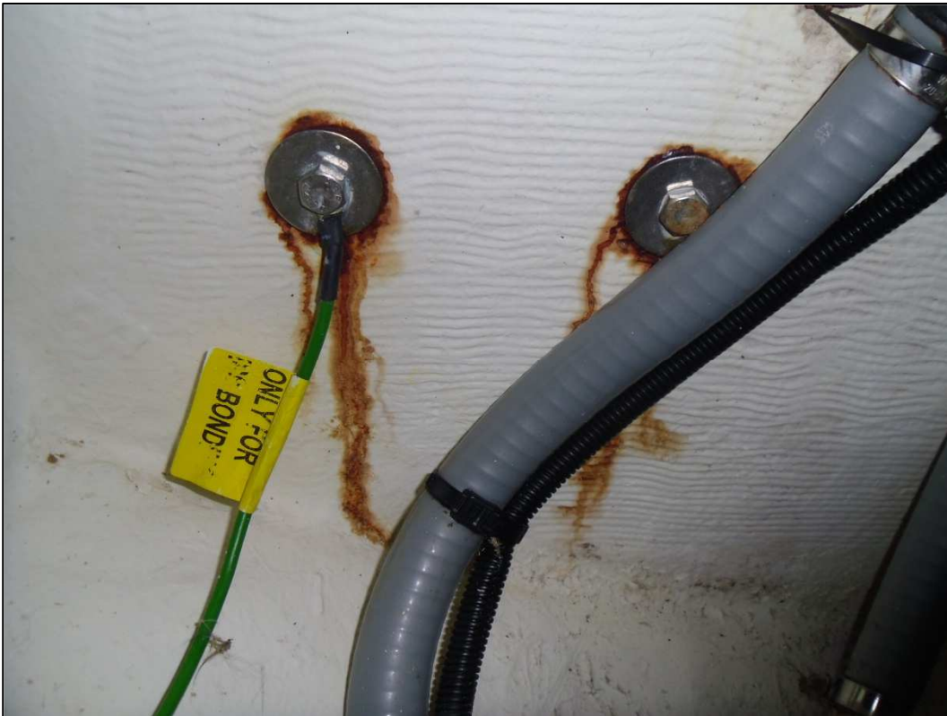
Fig.1 – evidence of leaks through some of the transom fixings.
