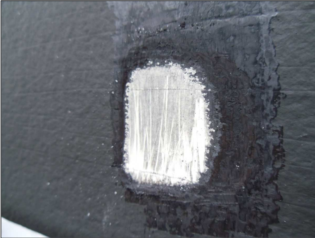
Fig.2 – stress cracks in the coatings and gelcoat.
