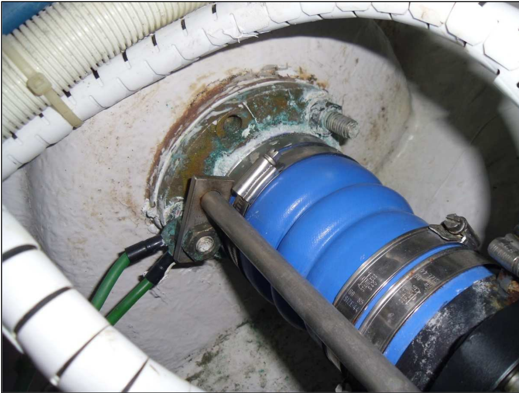
Fig.4 – salt deposits are evidence of a leak from the port stern gland.
