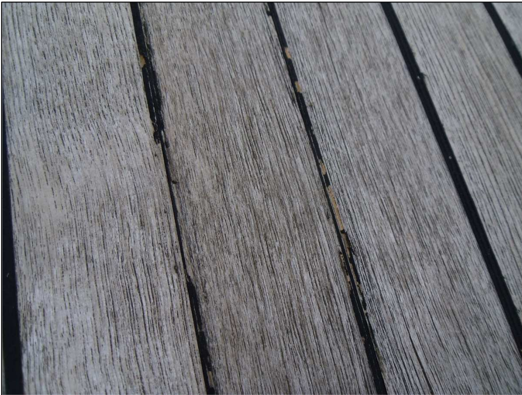
Fig.5 – teak decking showing areas of worn or missing caulking.
