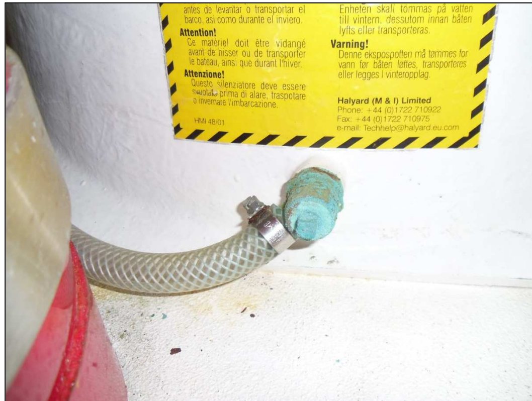
Fig.7 – corrosion to exhaust box drain connections.
