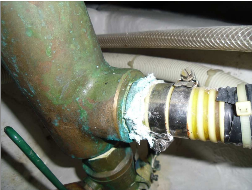
Fig.6 – air conditioning coolant seacock strainer outlet with salt deposits.
