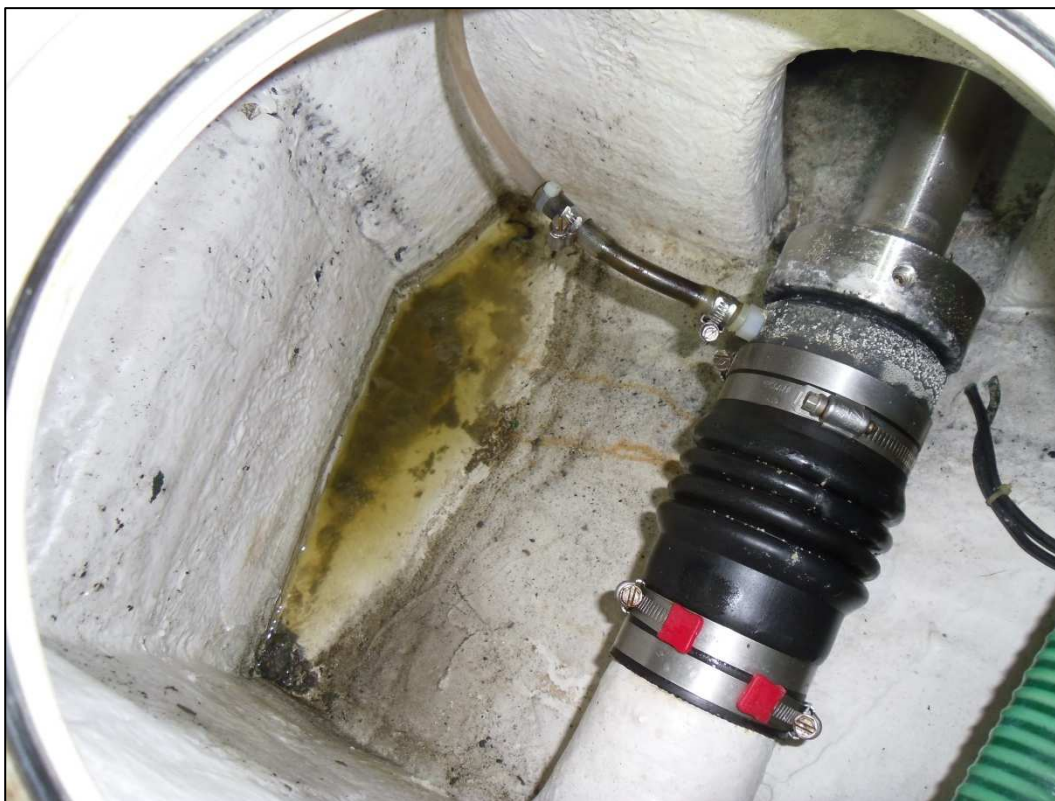
Fig.4 – starboard stern gland has a leak with long standing salt water in the bilge.
