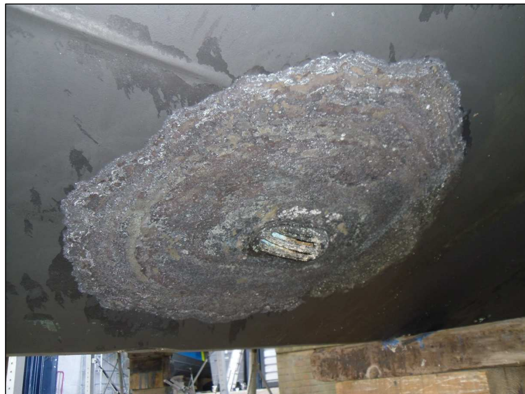
Fig.1 – Coppercoat blistering / reaction around skin fittings.
