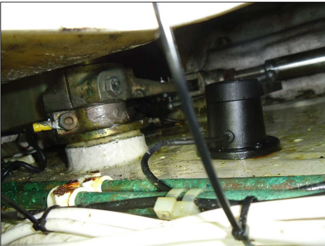
Fig. 6 – hydraulic copper pipes all showing signs of heavy patina / corrosion.
