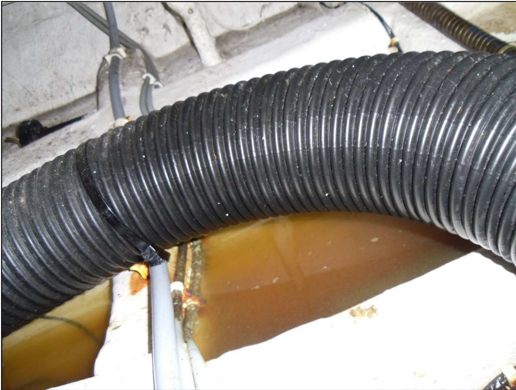
Fig.7 – areas of long standing salt water extreme aft and outboard on the starboard side.
