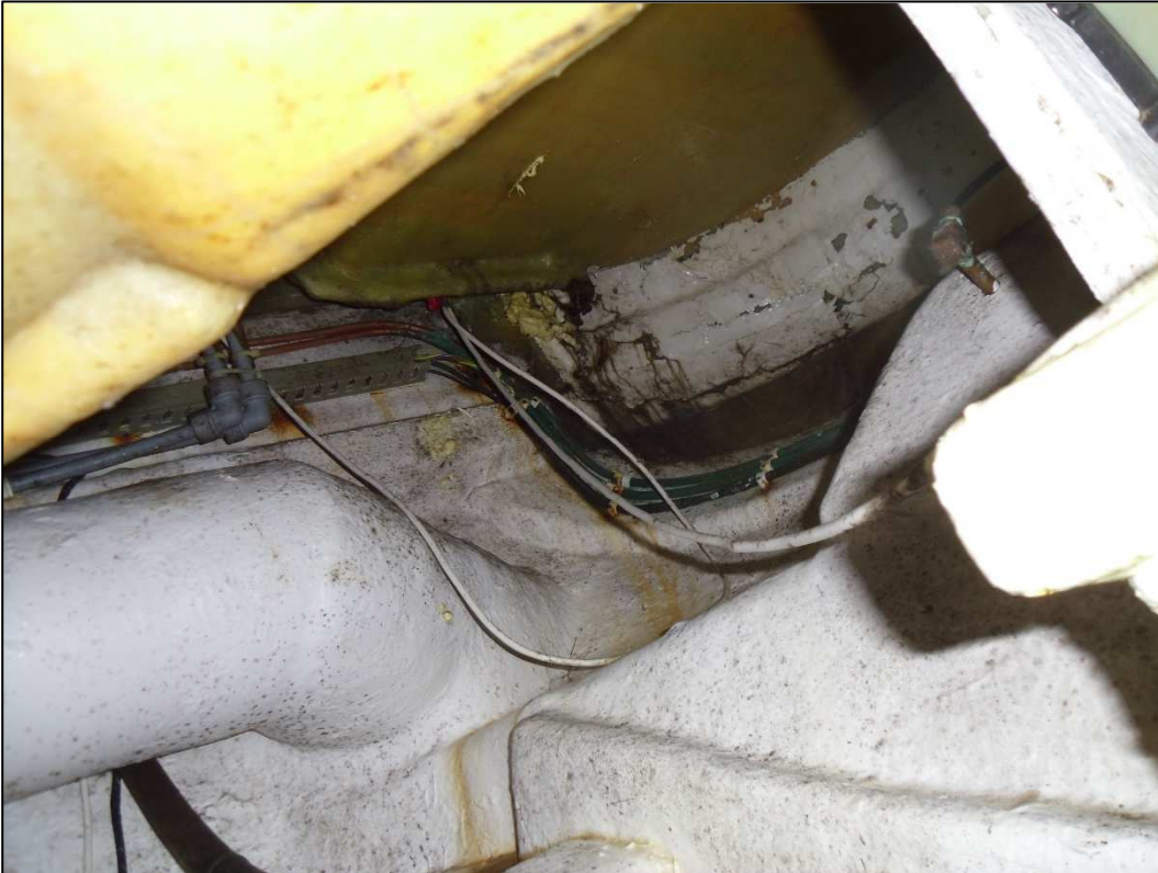
Fig.5 – various water leaks from the aft end / bathing platform on the starboard side.
