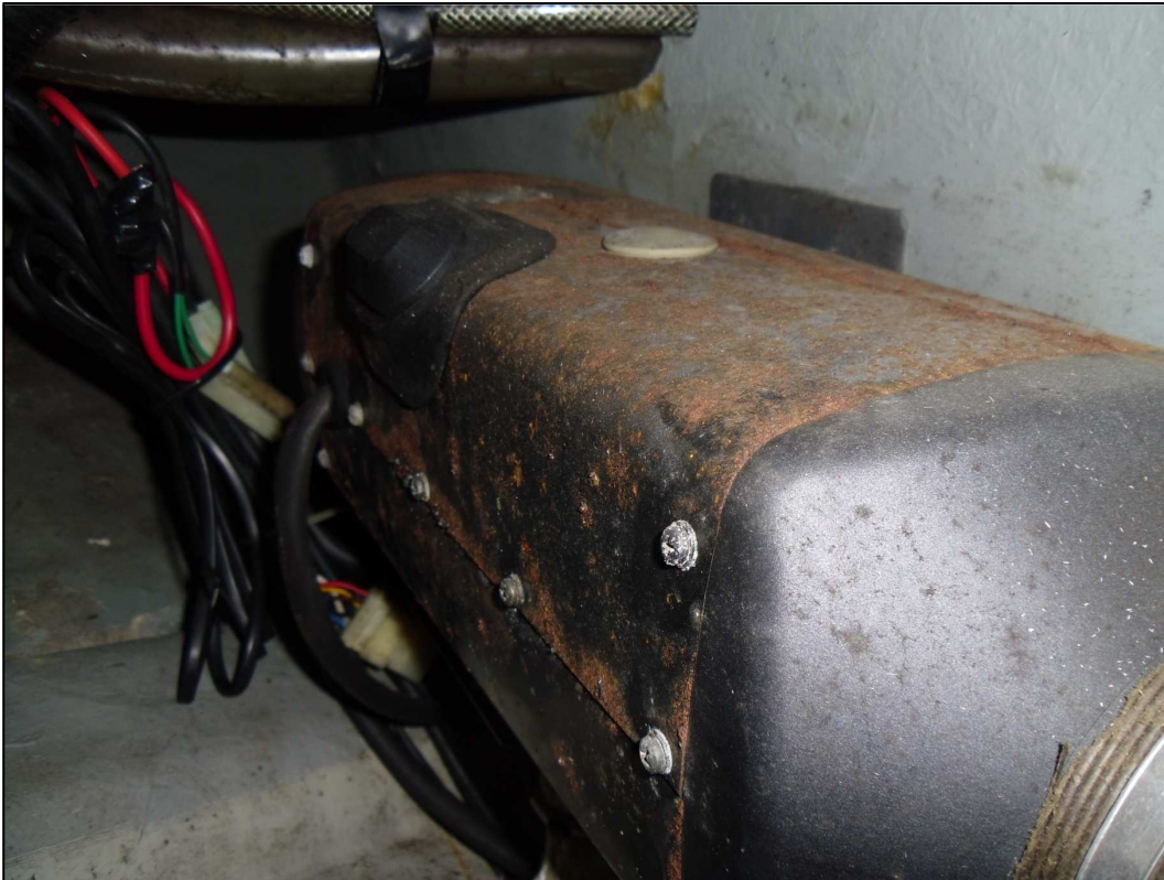
Fig.5 – diesel heater does not work and the casing is showing all over corrosion.
