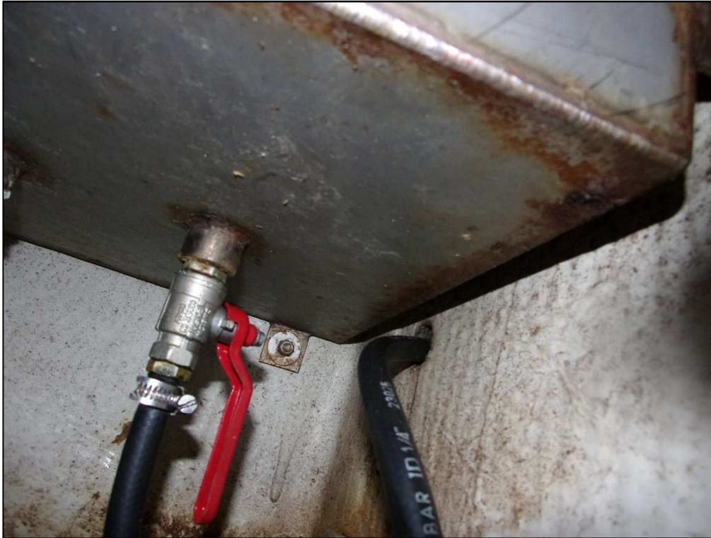
Fig.4 – the fuel tank cut off valve is very inaccessible in an emergency.
