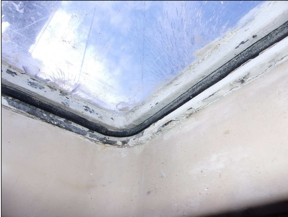
Fig.2 – poor hatch to deck head sealant showing leaks.
