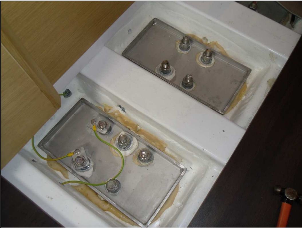
Fig.2 – keel bolts, fixings and backing plates.
